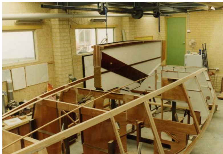
Bulkheads assembled on the building frame, chines and gunwales in place and the centrecase being lowered into position. Klaus noted that the chines were fabricated from two pieces of timber
