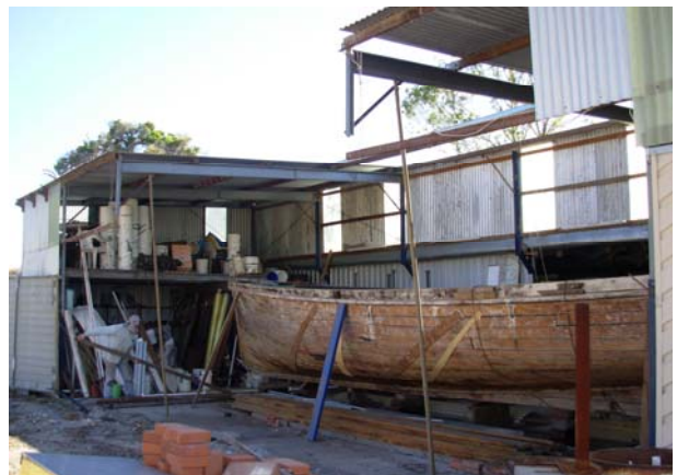
Kiewa's shed comes down for the second time to exit to Fremantle Boat Manufacturers 5/12/2007
